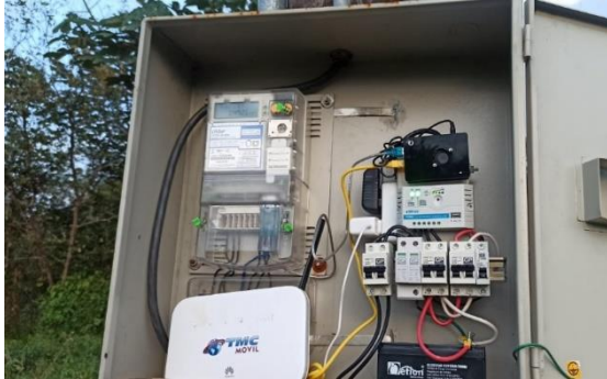
Fig. 5. Functional prototype installed in Mitú (Vaupés) Source: Own elaboration
