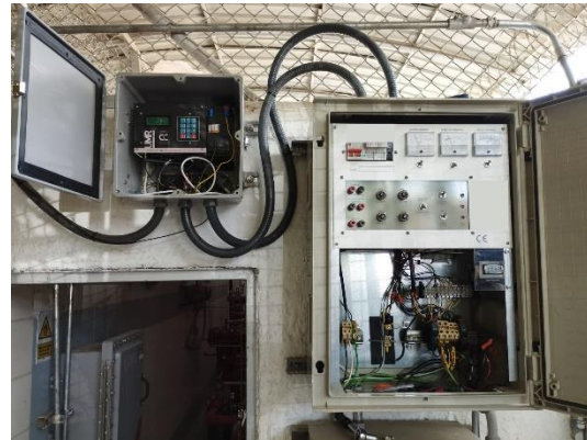
Fig. 10. RMU implemented on cathodic protection rectifier Source: Authors' own creation.
