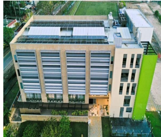
Fig. 1. Photovoltaic solar plant located on the roof of the building.
