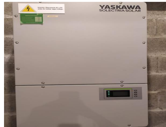
Fig. 2. Solar inverter No. 1 of the plant.
