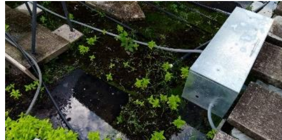
(c) Water valve box.
