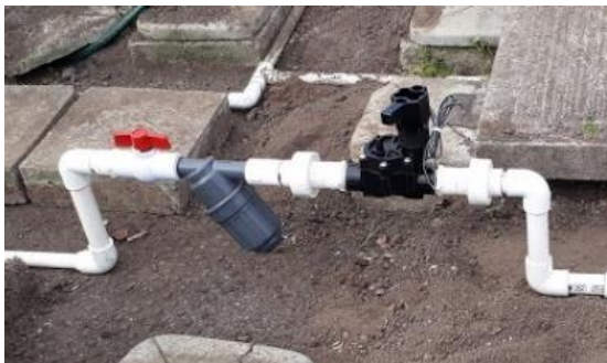
(b) Water pipe ball valve, water filter, and water electro valve.
