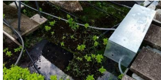
(c) Water valve box.
